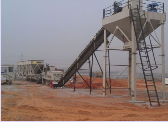
WET MIX MACADAM PLANT
